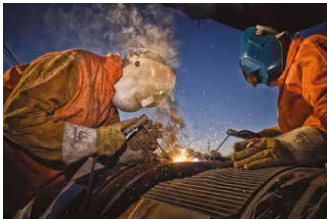
Figure 6. SMAW front-end welders applying the vertical-down hot pass, at top of pipe.
