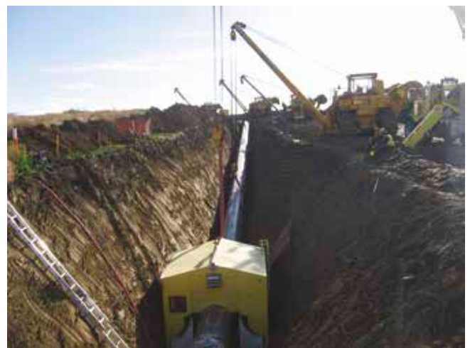
Figure 11. A shack being prepared for mechanised welding of a ditch tie-in joint.
